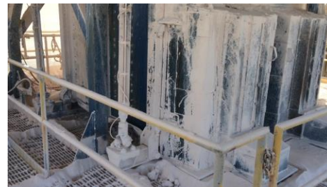
Figure 2—Vibrating screen causing resonance in a structure
